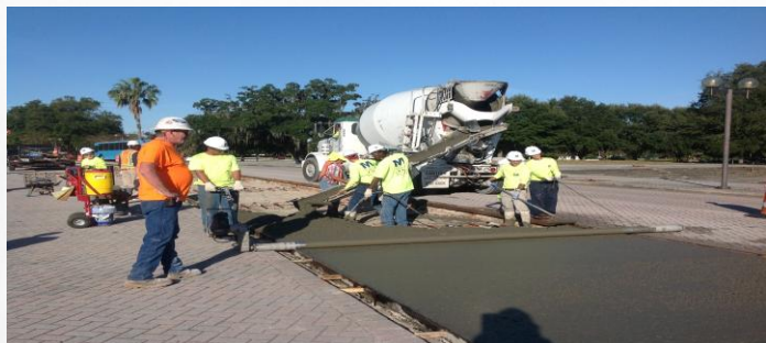
Amelia Street: Crews using a rolling screed to finish the new concrete turn lane.
