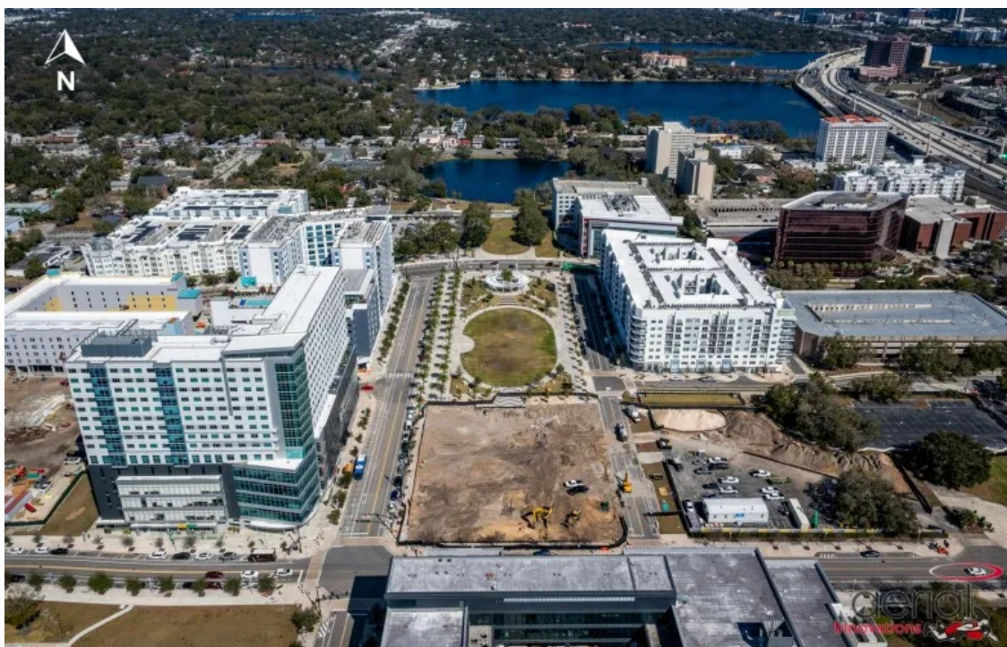
This aerial image taken on Feb. 19, 2026 shows the construction site of the Parcel H building south of Luminary Green Park and The Beacon just west of The Julian apartments. (Courtesy of Ustler Group of Companies)
